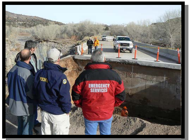
Washington County Emergency Manager Peter Kublmann with the State of Utah's Hazard Mitigation Officer, Brad Bartholomew, and FEMA representatives surveying damage and repairs to a bridge north of Gunlock
